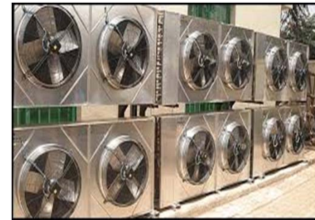
Service sector cooling
