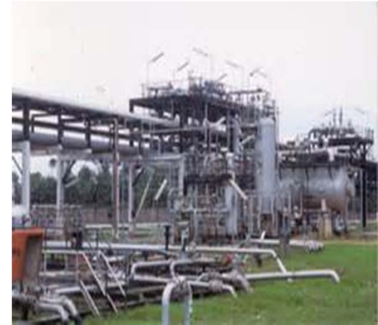
Nigeria gas production facility ( sweetcrudereports.com )
